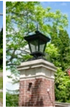
.35, .36 Entrance Gate Structure with brick and stone detailing and lanterns at the primary gate posts.
