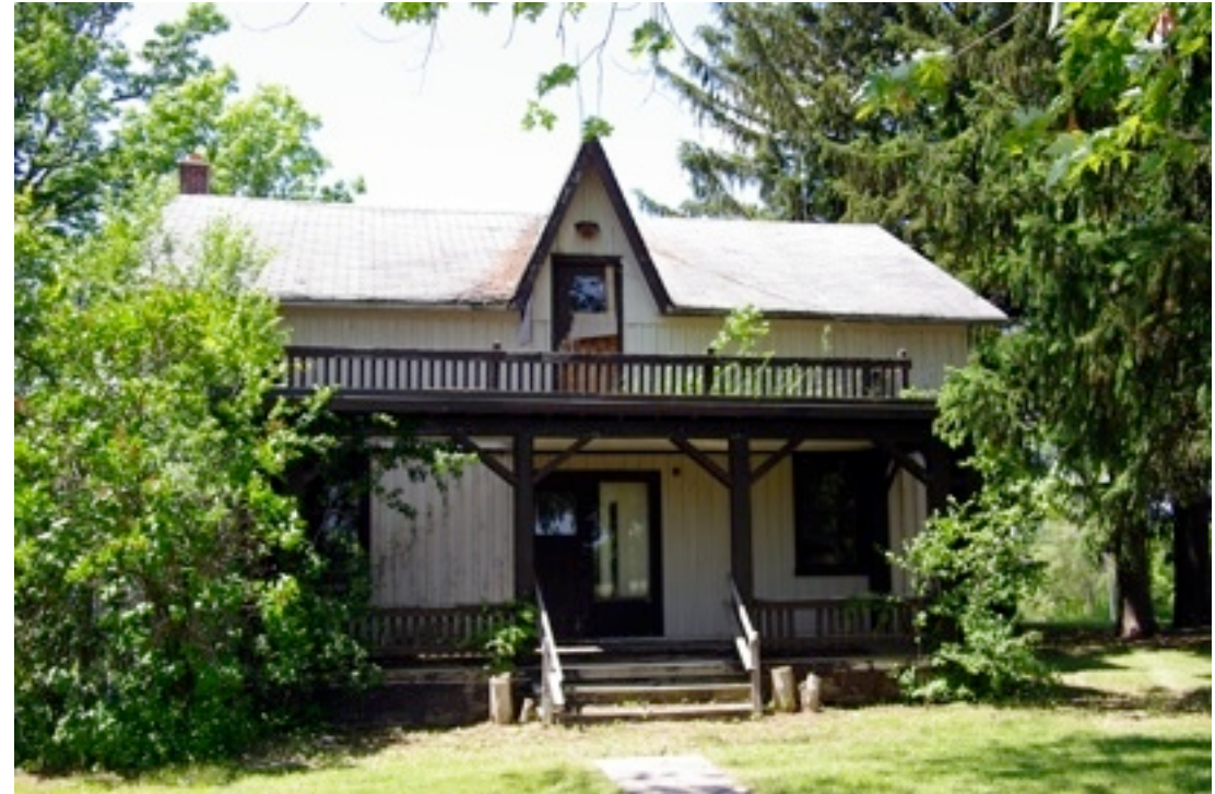
.6 The Ferguson House c.1850s. This is a view of the front, east elevation, and shows that the form and most of the original design is intact. Some or all of the porch may have been altered and the windows and doorway have been replaced in the original openings.
