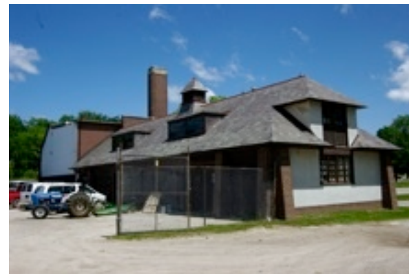
.11, .12, .13 Front wing of the dairy farm. The original use of this wing needs to be confirmed but it would appear to be cattle stalls to the left and a head “office” building to the right. Note that the roof line is altered from the 1920 appearance. this may reflect repairs after the less serious fire in 1937.
